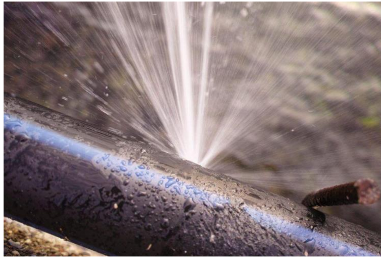
Figure 1 Image of a pipe burst anomaly.
